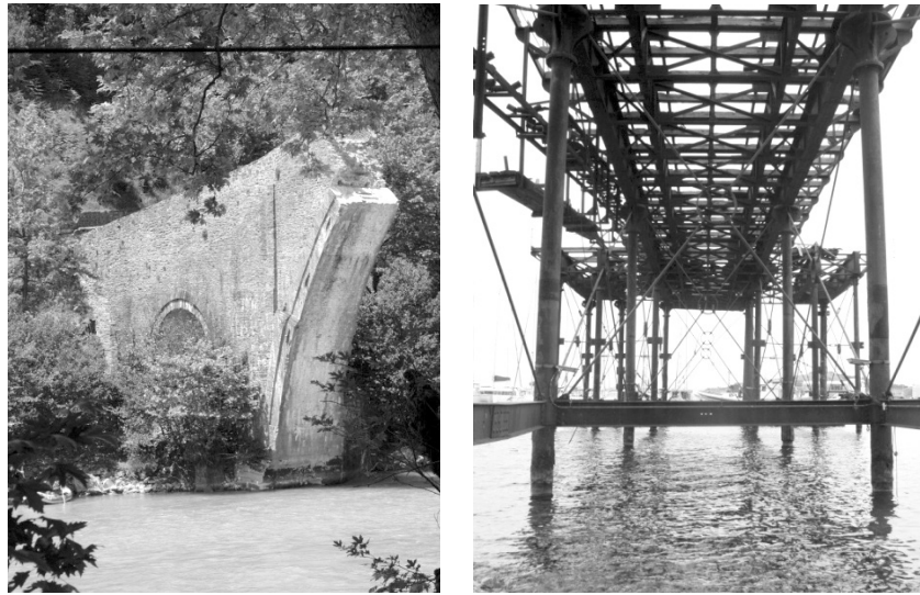
Fig.4: left: the stone bridge of Plaka in Epirus, right: French wharf in Lavrion
