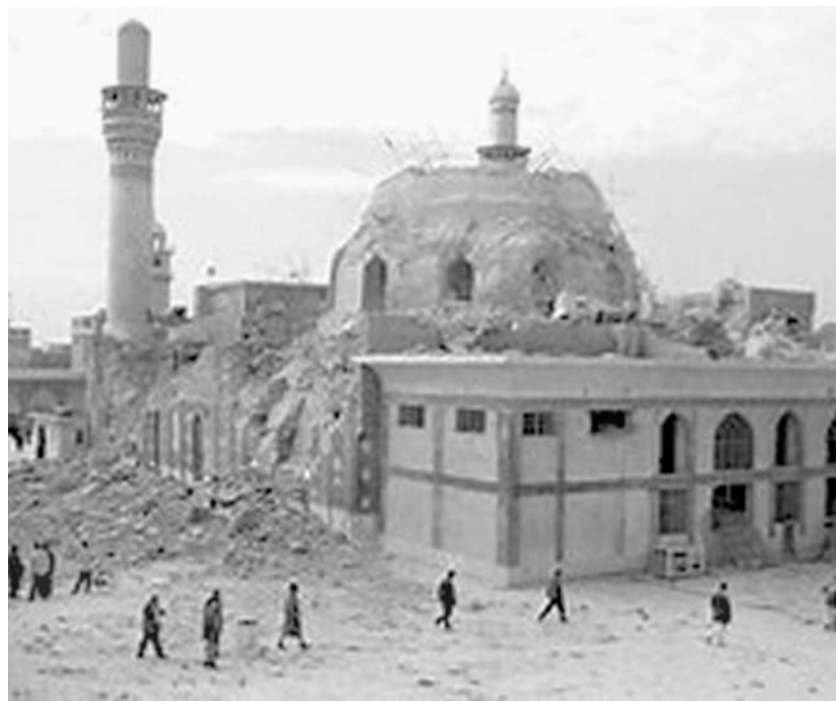
Fig.2: The extensive damage to the al-Askari Shrine in Samarra, Iraq has been regarded by many as the tipping point that turned general unease with the Coalition presence in Iraq into a full scale, sectarian, civil war. Photo: © US Army, via Wikimedia Commons.
